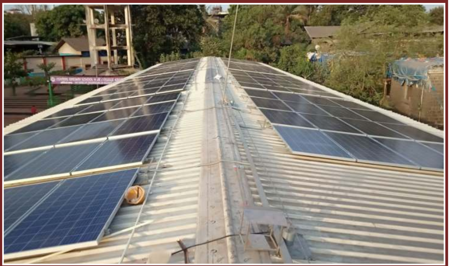
50 KW ON-SITE SOLAR PV UNIT INSTALLED ON SCIENCE BLOCK
