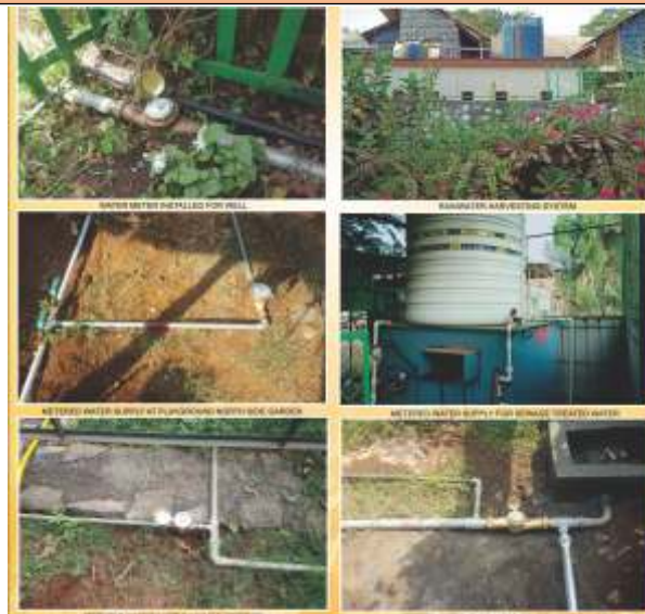
WATER METERS INSTALLED IN CAMPUS
